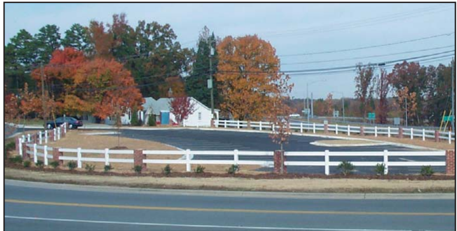
Inviting park-and-ride lots are an essential element of improving regional transportation. Thomasville site nearing construction completion.
